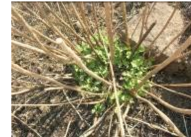
Vegetation grown in cracks of basalt
