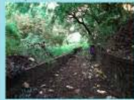
Condition of internal road, no access over there, road act as a dump area.
