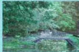
Bridge covered by full of trees and shrubs, no access over there.
