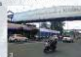
A over bridge is constructed for the crossing from the parking area to the Garden.
