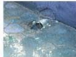
Storm water drainage problem
